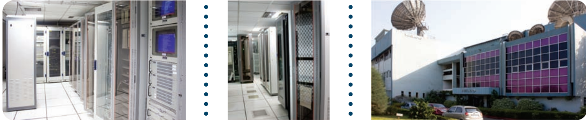
Tatanet's new Datacenter facility at Nelco H.O, Mahape
